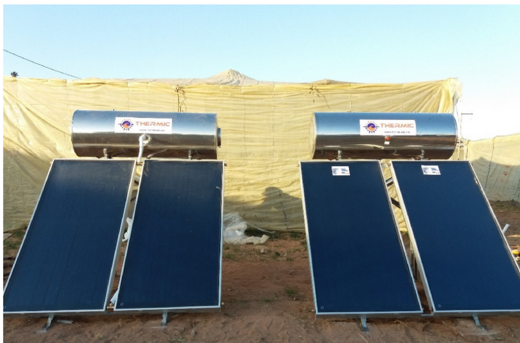
Fig. 2. ThermoSiphon thermal solar collectors with water closed-circuit and 300 L of storage volume.
